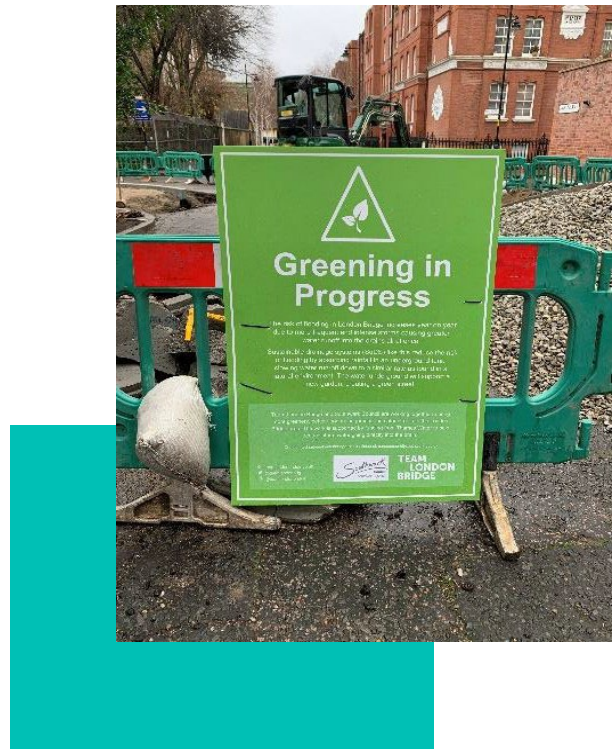
Figure 3-2 Photograph of works notice for the London Bridge SuDS Scheme at Melior Street (Credit: Southwark Council)
